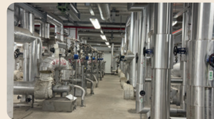
Improvement of heat transfer system
